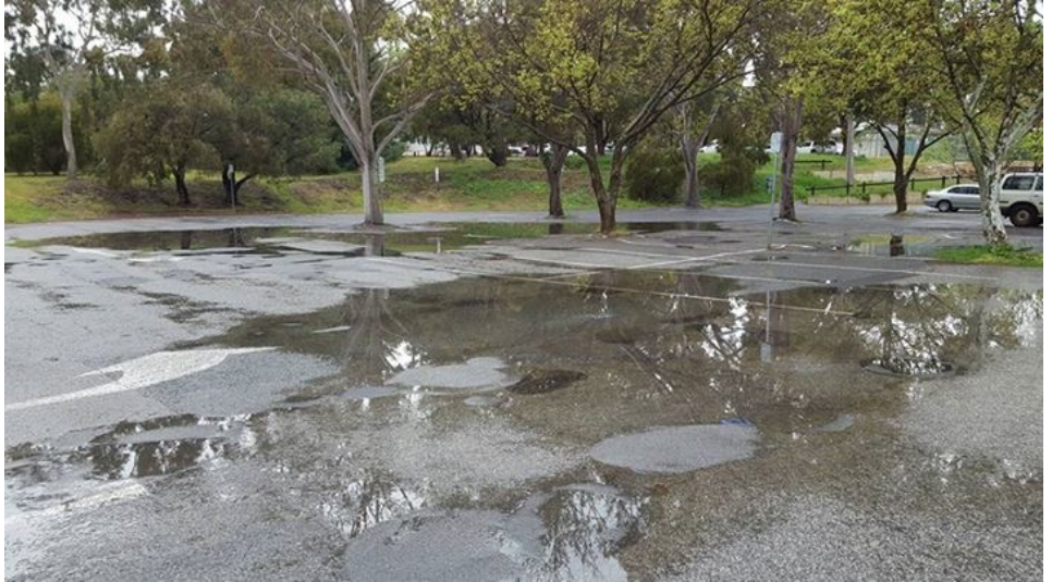
A very wet car park!
